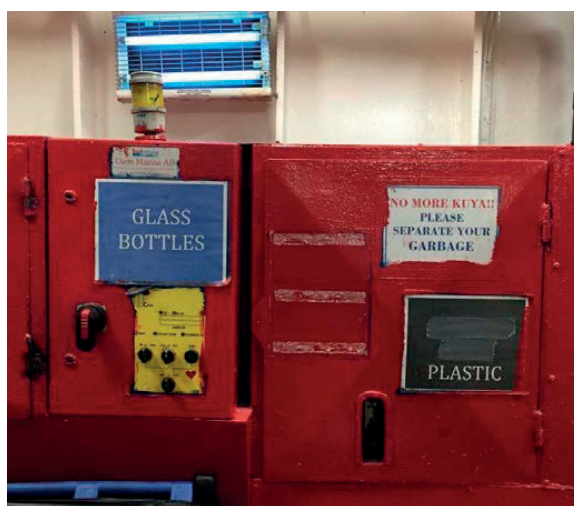
Garbage room and compactor. Source: Australian Maritime Safety Authority
