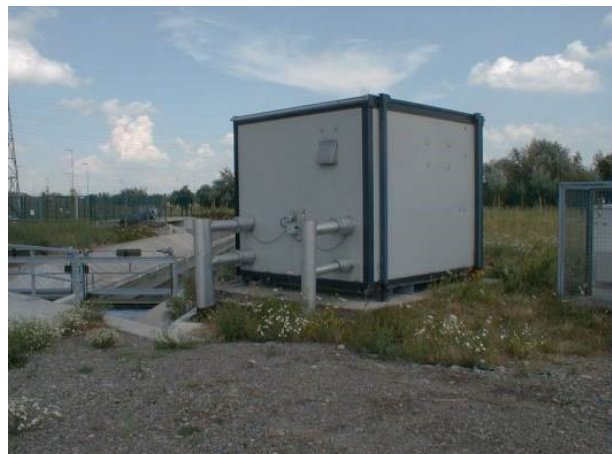
outside container view
